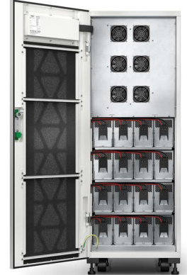
40kVA Easy UPS 3S with internal batteries
